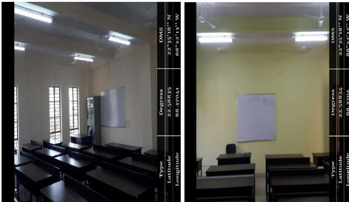
LED LIGHTS IN CLASSROOMS
