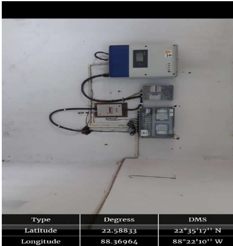
SOLAR METER THROUGH WHICH SOLAR ENERGY IS WHEELED TO THE GRID
