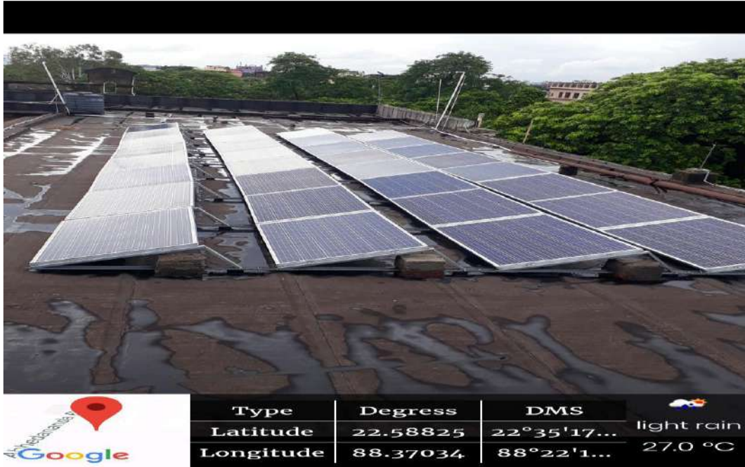
SOLAR PANELS ON ROOFTOP
